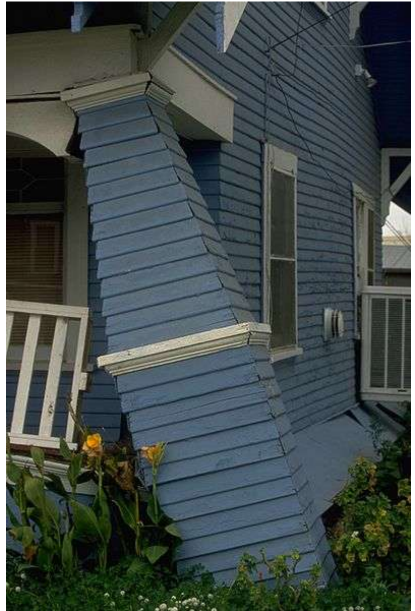
Fallen Decorative Work.
