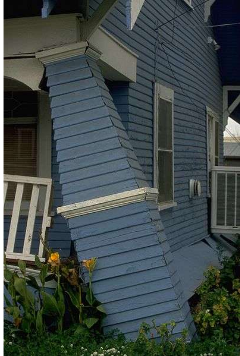
Fallen Decorative Work.
